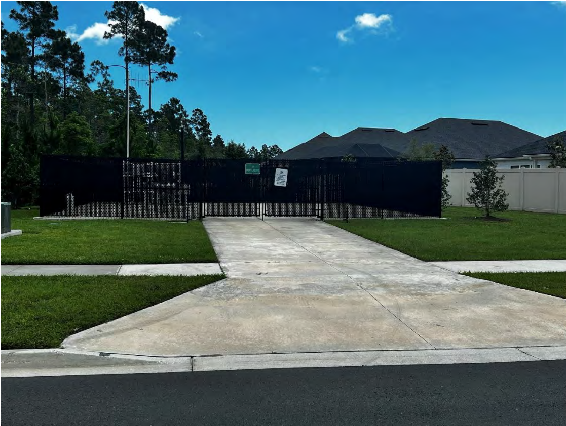
Trophy Lake Drive Lift Station (05-21-2026)
