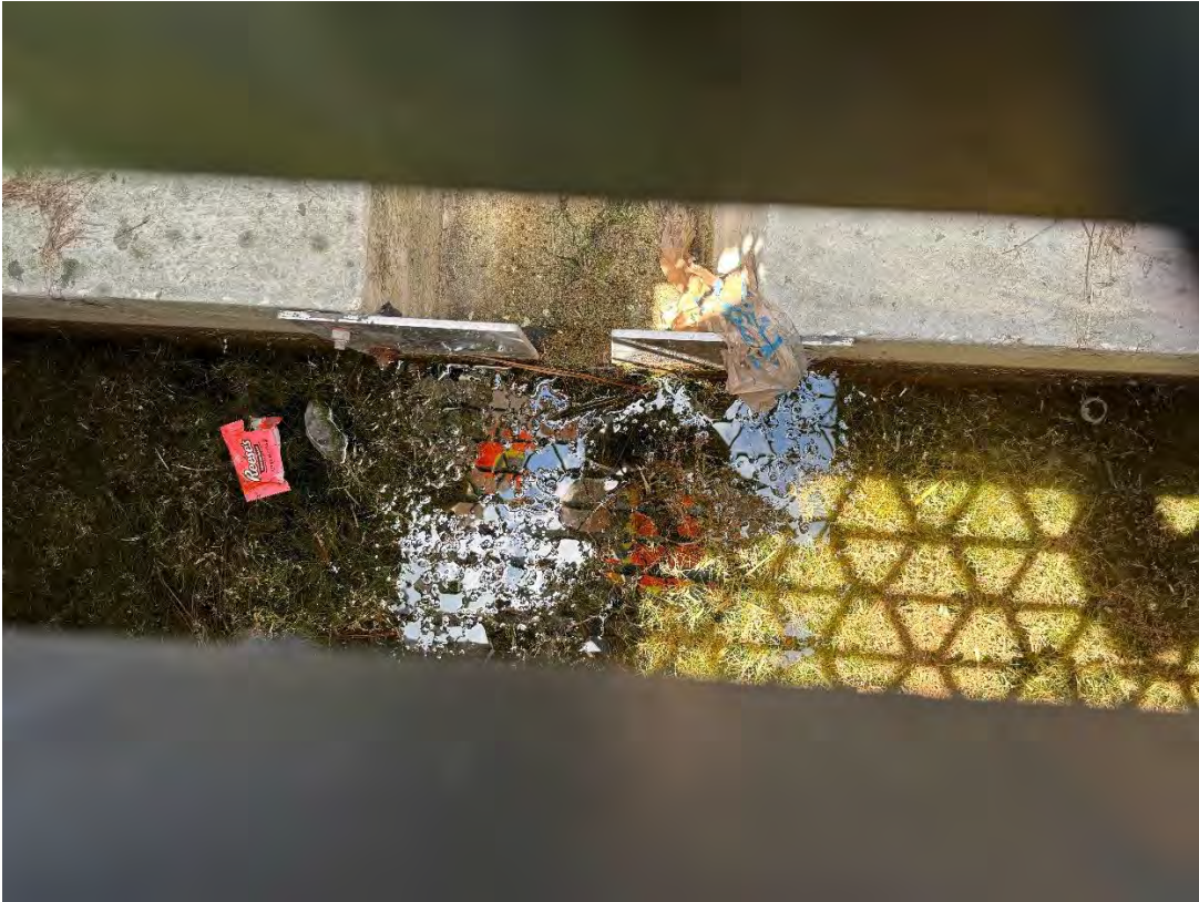
Beacon Lake Phase 2C – SMF 20 Waste & Debris in Control Structure (05-21-2026)
