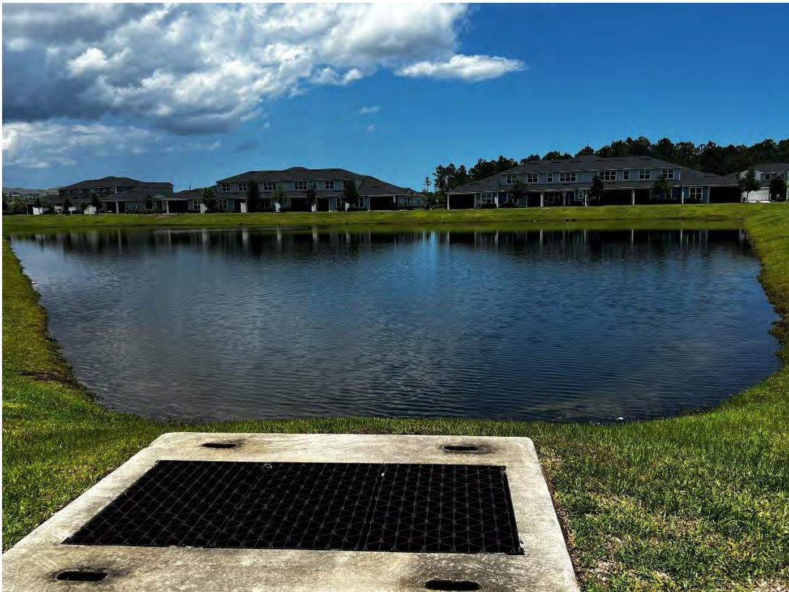
Beacon Lake Townhomes – SMF 10 Control Structure (05-21-2026)
