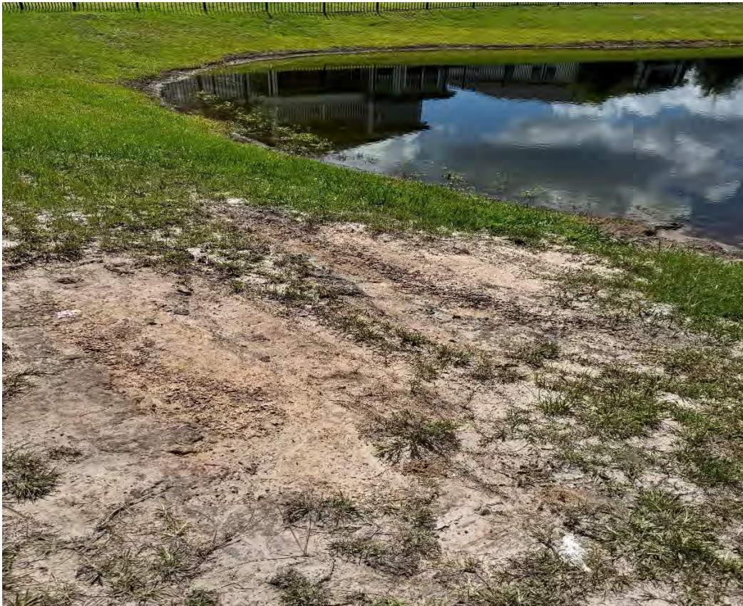
Beacon Lake Phase 2C – Erosion & Disturbance on SMF 20 Bank, Tire Marks Visible (05-21-2026)
