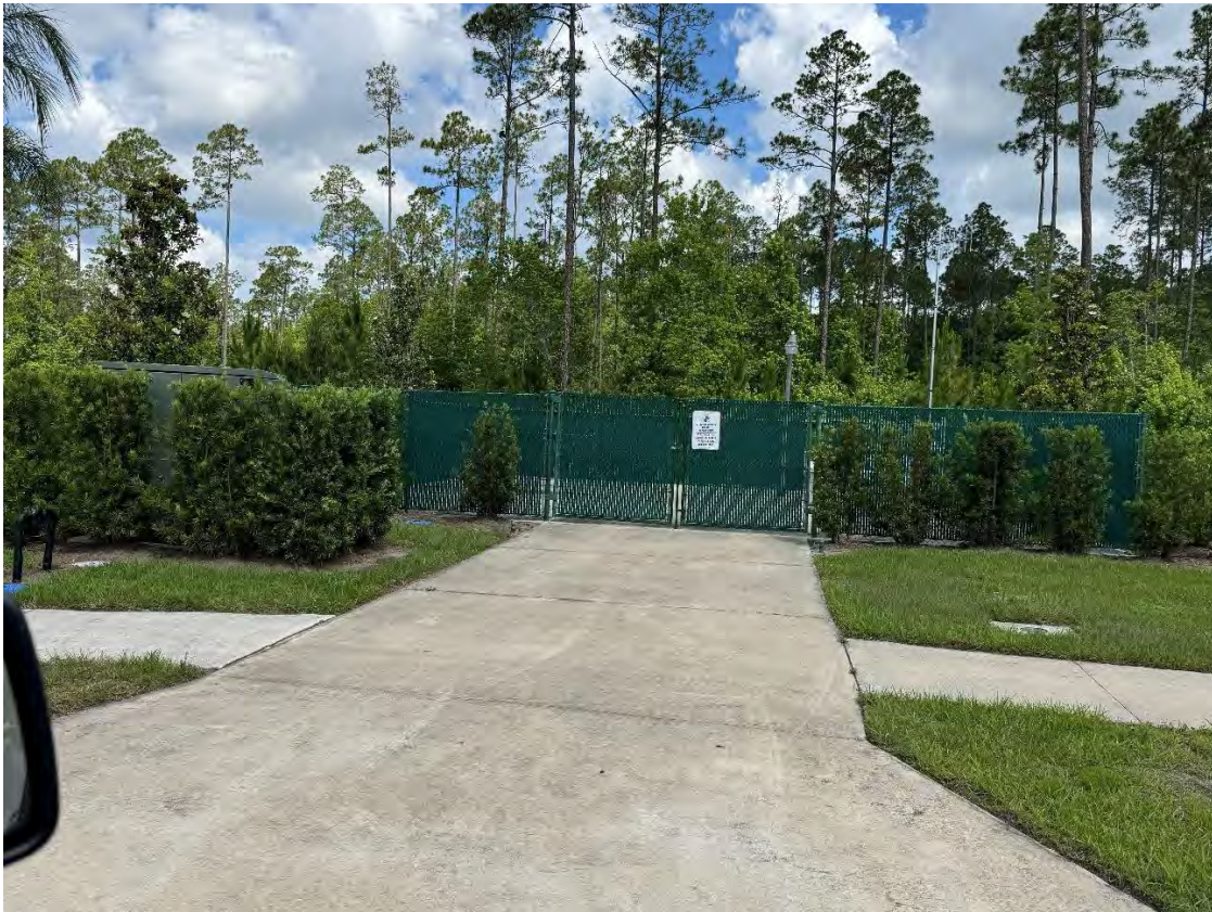
Windermere Way Lift Station (05-21-2026)
