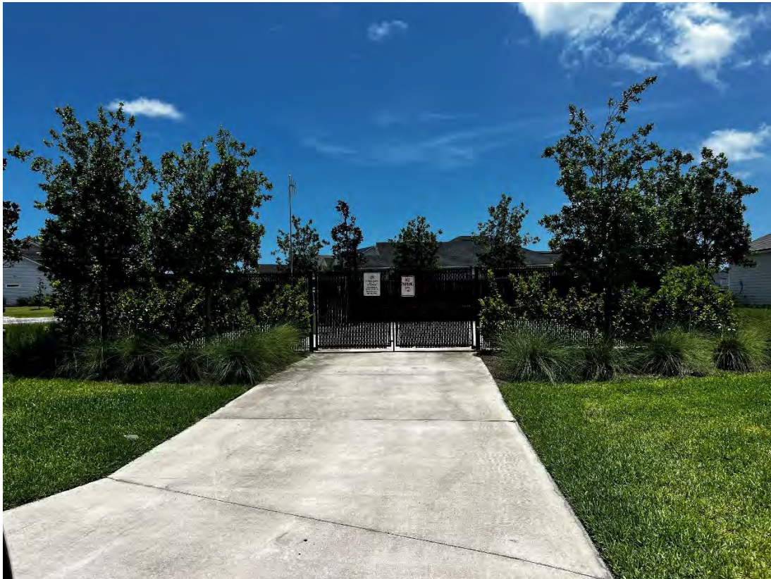
Whirlwind Place Lift Station (05-21-2026)
