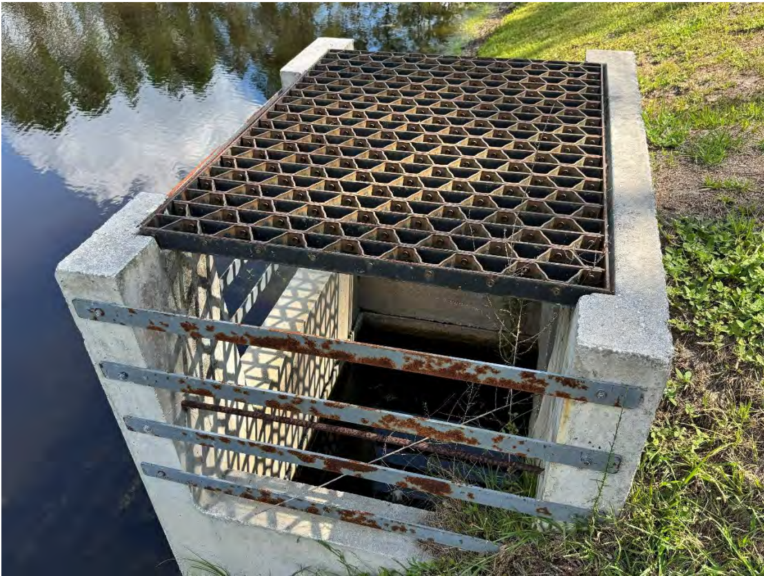
Beacon Lake Phase 1 – SMF 4 Control Structure (05-21-2026)
