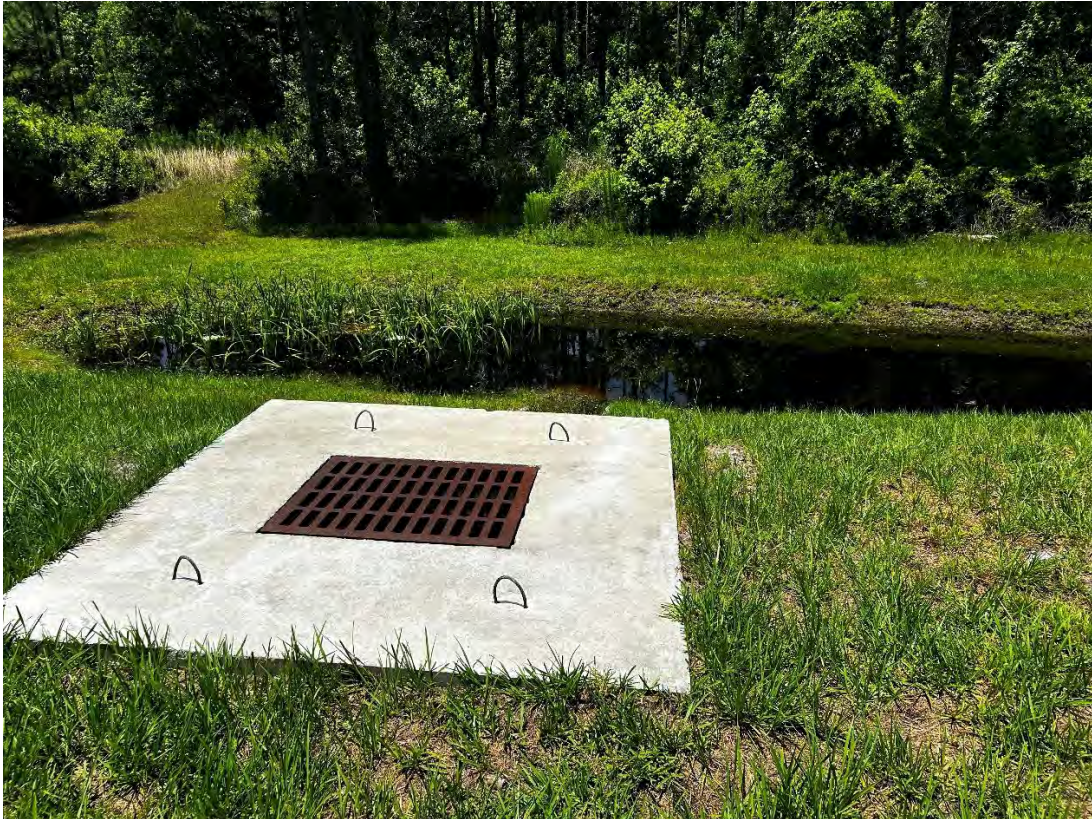
Beacon Lake Phase 4 – SMF 23 Control Structure (05-21-2026)
