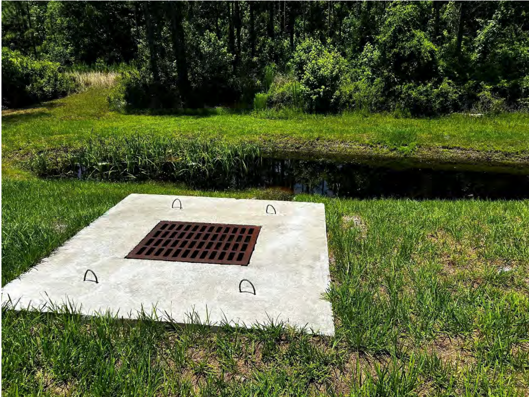
Beacon Lake Phase 4 – SMF 23 Control Structure (05-21-2026)
