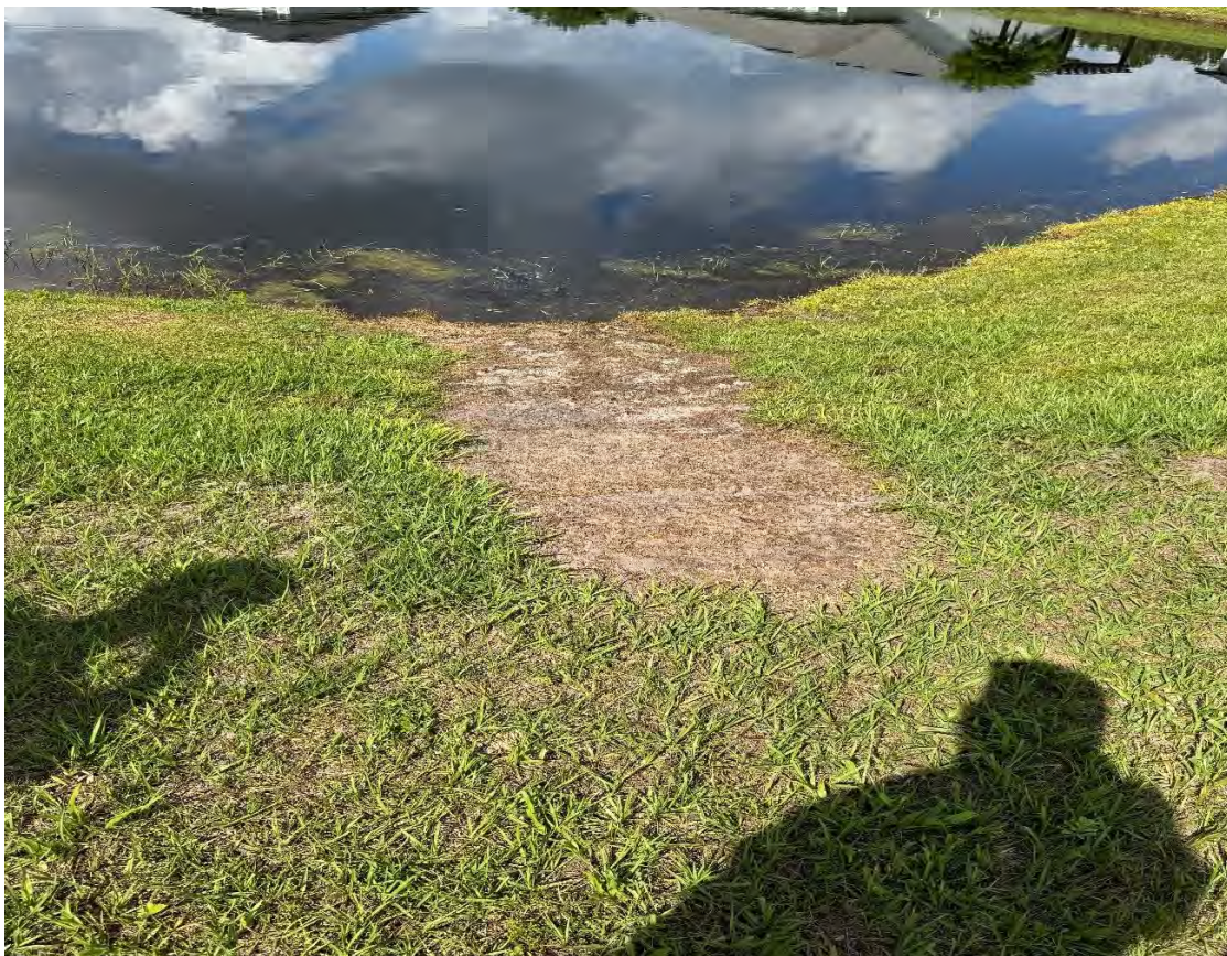
Beacon Lake Phase 1 – SMF 13 Washout/Erosion (05-21-2026)
